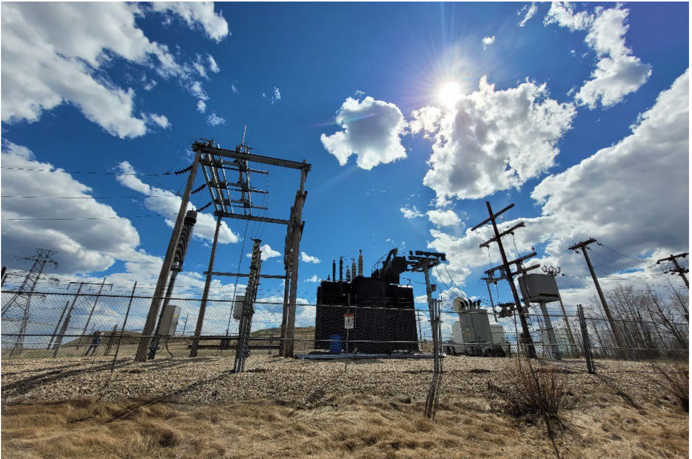
Existing AltaLink Substation Marion 21S Substation
